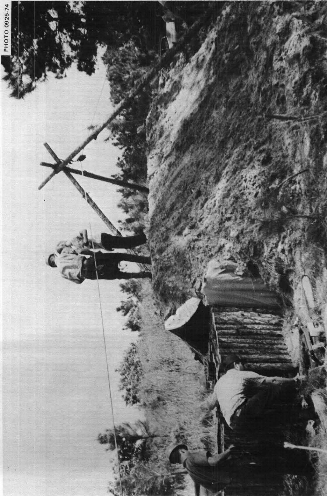
Fig. 5.51. The pulley conveyor system actually wasted energy and time, since earth had to be lifted in a 5-gallon paint can up to the hook on the movable pulley; then the earth-filled can was pushed up the upward-sloping nylon rope to a position several feet above the top of the shelter. Then most of the earth rolled down below the top of the shelter, obviously wasting thousands of foot-pounds of work.
